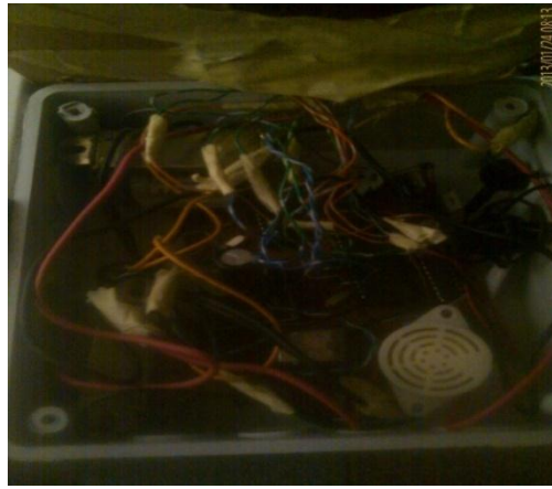
Interior view of the controlling unit
