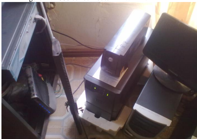
Figure 5i: SMART iWLAN server room devices
