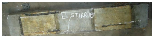
Fig 4.4 Failure of beam N-SB1
