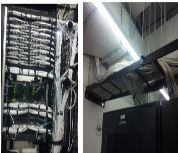
Figure 3: A Switch Closet of a Small Company. The left side picture shows the main switch rack with huge bundles of cables intertwined with each other. The right side picture shows the huge bundle of cables going to riser channels and lateral ceilings from the rack.
