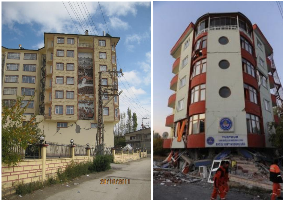
Figure 6 Damage to unsymmetrical irregular structure
