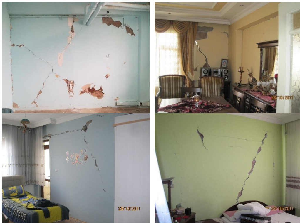
Figure 4 Excessive damage in brick infill walls
