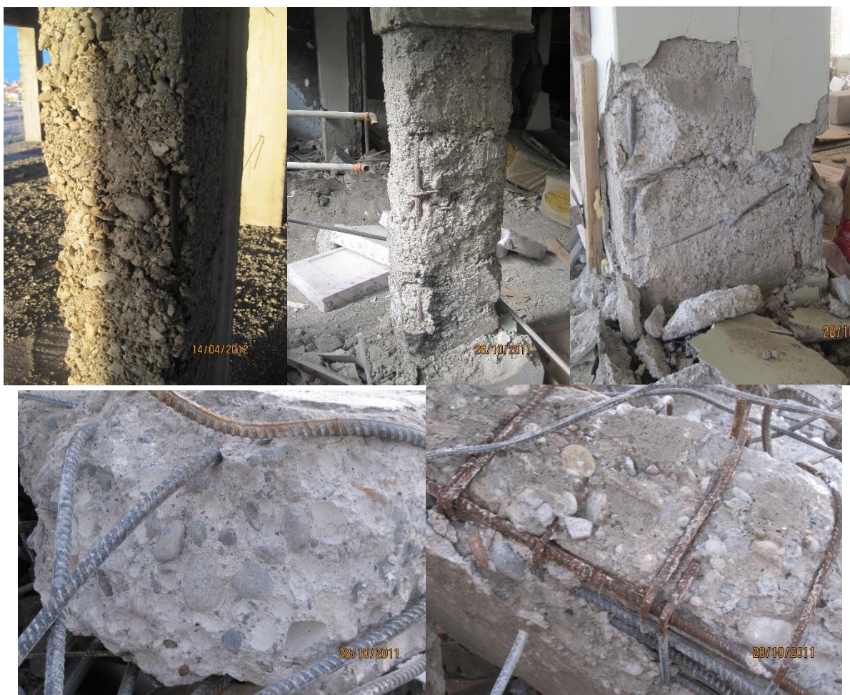
Figure 12 Concrete material condition in RC buildings
