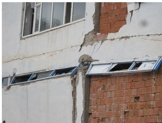
Figure 11 Short column failure
