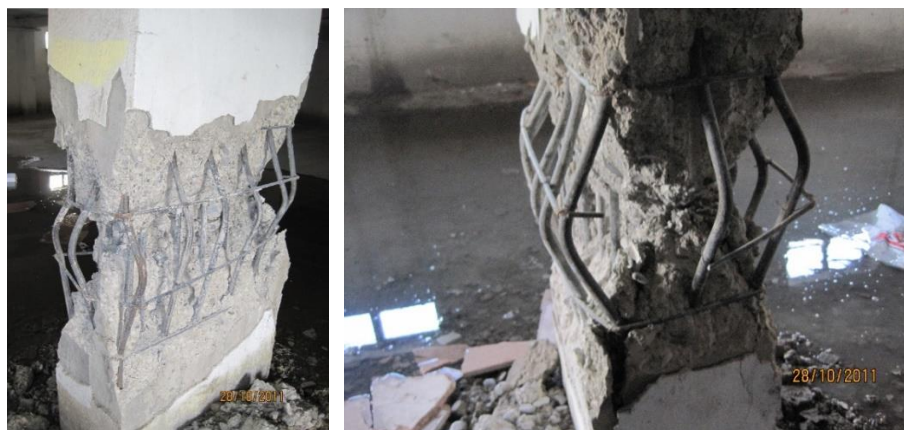
Figure 8 Buckling of longitudinal reinforcements
