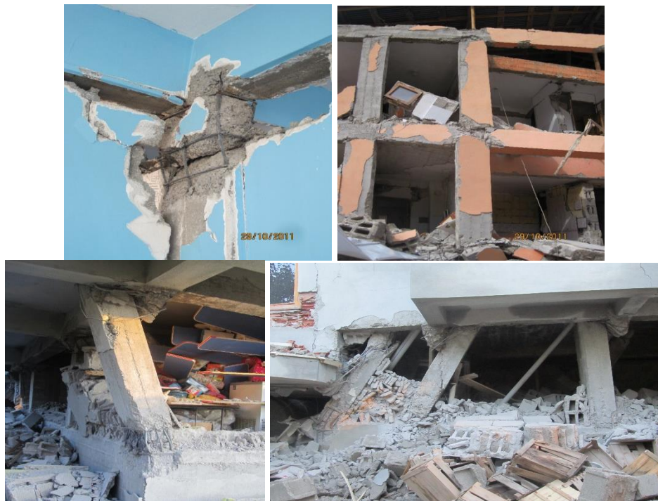
Figure 9 Failure of beam-column joints
