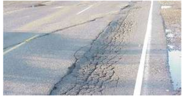
Fig.3. permanent deformation (rutting)
